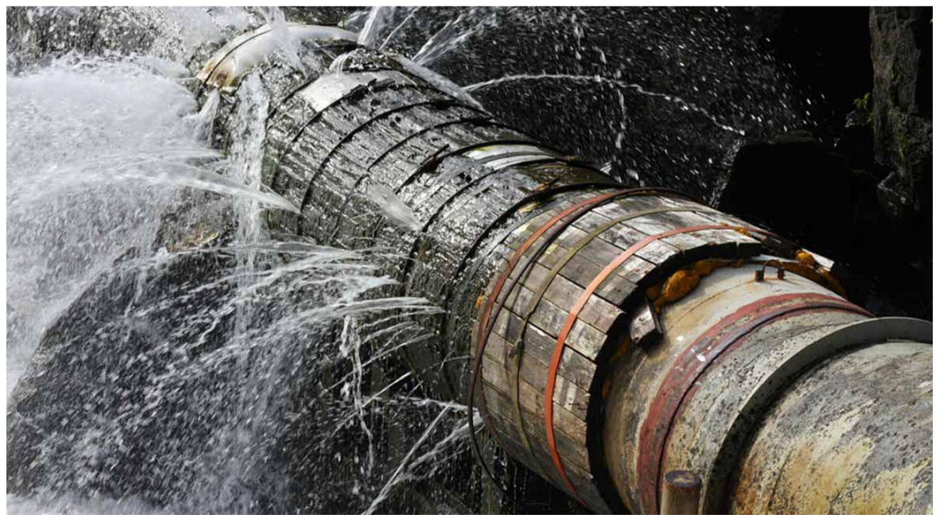
Computers can help to combat water shortages by monitoring the infrastructure.
